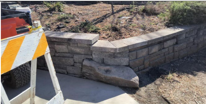
Figure 3. The wall at the TARC after being fixed by maintenance.
