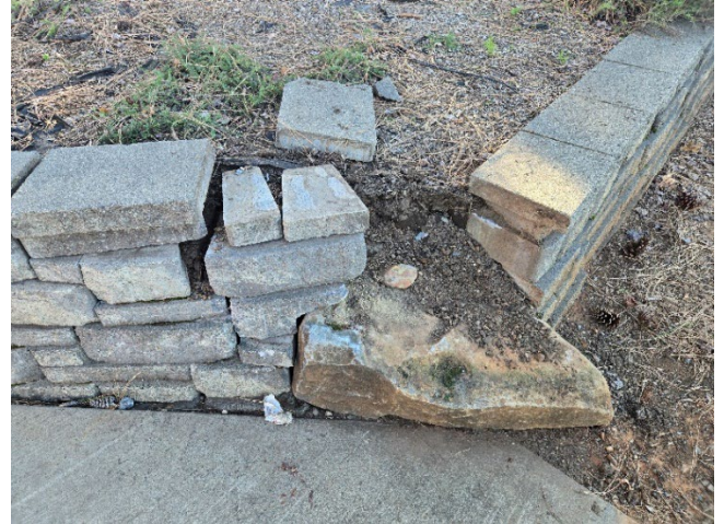
Figure 2. The wall outside the TARC that was damaged by a car crash (before).
