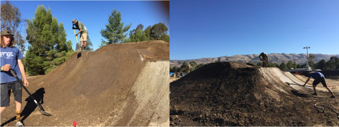
Using shovels to pack and shape dirt jump lip. Using the concrete kicker to shape to.
