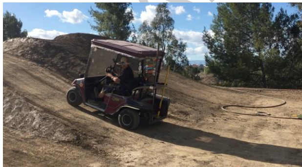
Using a push broom to smooth out the jump lip and prep for final compaction. Final compaction with golf cart.
