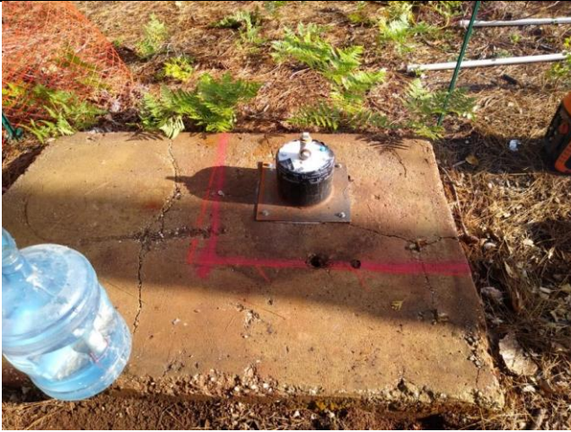
Figure 13. Old well pad
