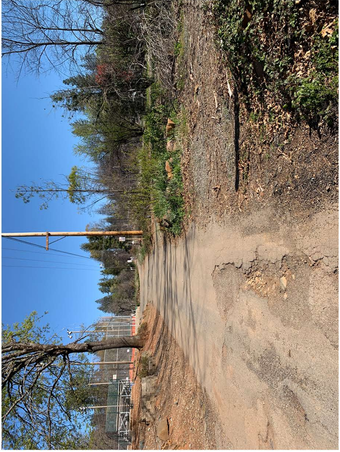
MOORE ROAD - NEEDS REPAIRS
