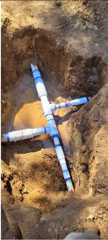
Figure 9. Maintenance fixed a broken pipe in the middle of the horse arena.
