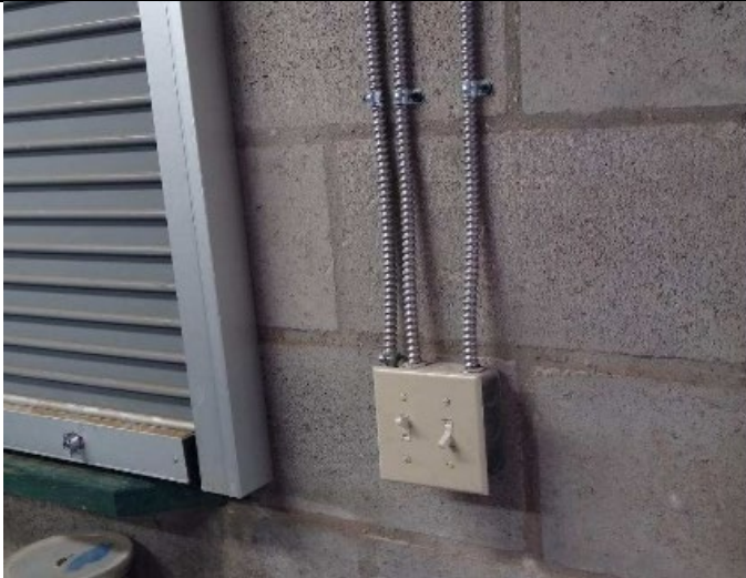
Figure 7. Maintenance added wall switches in the score booth at the horse arena for the lights/
