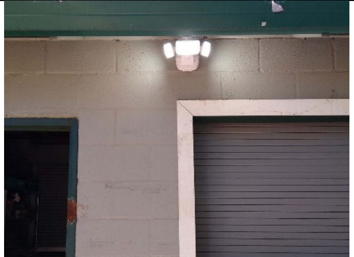
Figure 8. Maintenance staff added new lights to the outside of the building at the horse arena.
