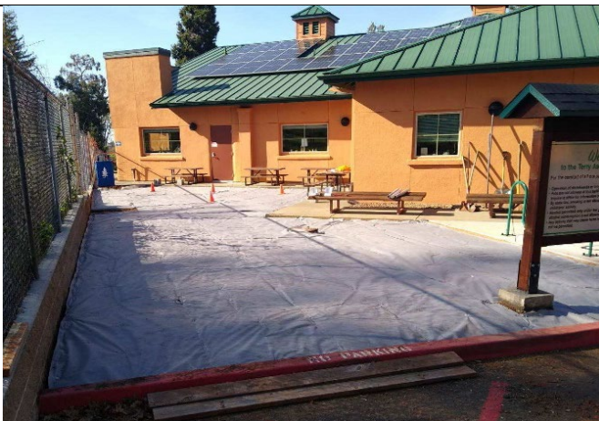
Figure 5. The maintenance crew removed the bark at the TARC and replaced it with rock.
