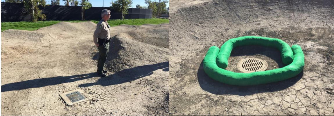
Winterizing drainage inlets with straw waddles and filter fabric will ensure they don't clog or release sediment into the storm water system.
