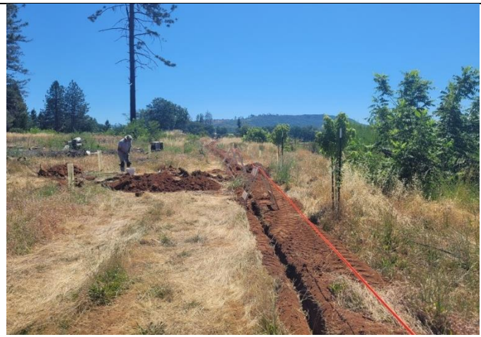
Figure 6. Maintenance staff digging to put in new irrigation lines at Noble Park.
