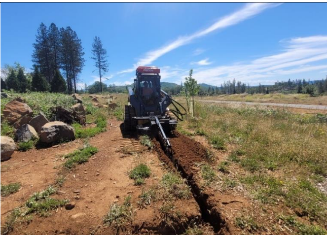
Figure 5. Maintenance staff digging to put in new irrigation lines at Noble Park.
