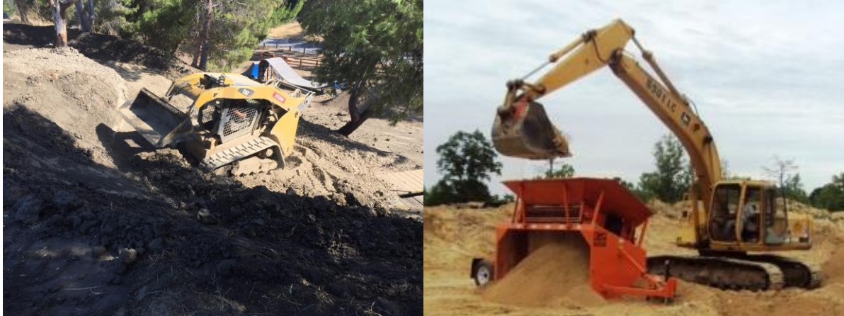
Conditioning a larger work area with a skid steer. Conditioning a soil stockpile with an auto sifter.
