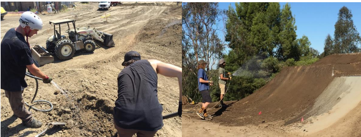
Workers processing materials mixing soil and water together and continue to moisture condition throughout the process to ensure good compaction.
