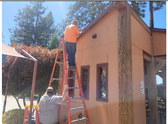
Figure 4. The Maintenance Crew is starting to repaint and stain the TARC. The BBQ area before.
