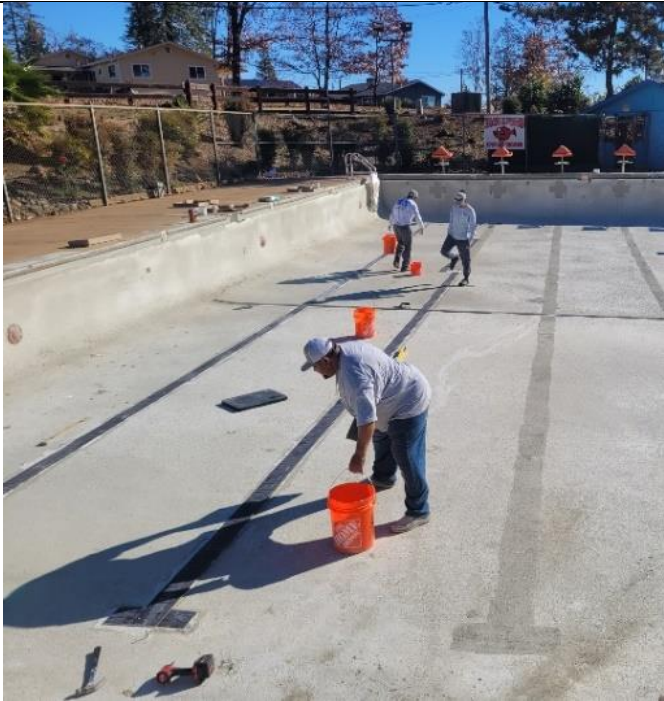
Figure 3. Maintenance workers lifting the tiles on the pool floor before the lining is redone.
