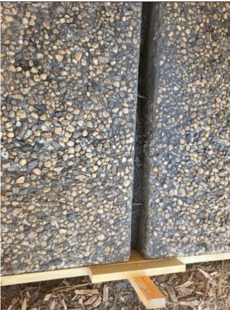
Figure 11. Expansion joints on path at Bille Park (before).
